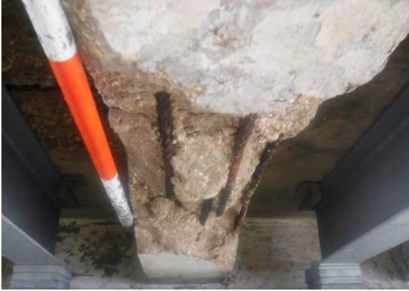
Figure 4.5 Reinforced Concrete Beam Damaged by Rebar Corrosion
