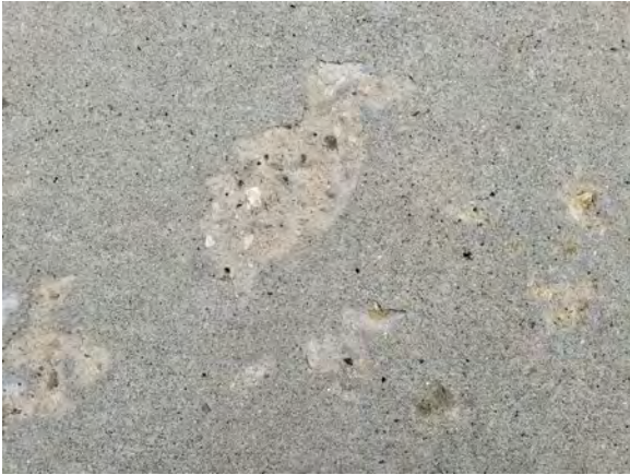
Figure 4.3 Concrete Scaling Damage
