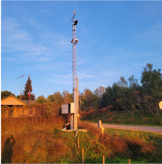
Figure 8.1 Typical Road Weather Information System (RWIS) in Wisconsin
