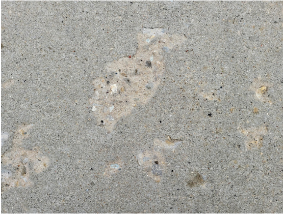
Figure 4.12 Concrete Scaling Damage
