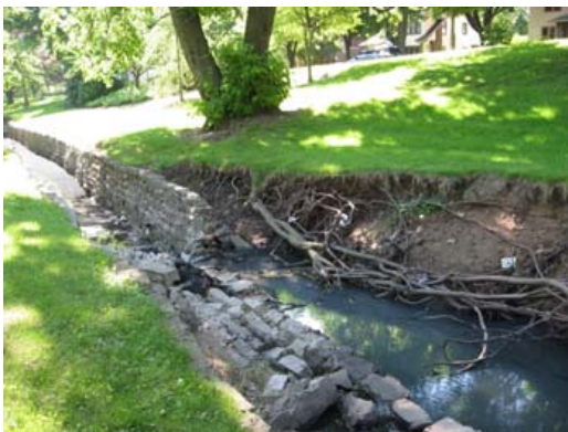
Bank failure along W. Lloyd St.
