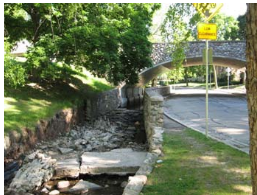
Channel erosion just south of Washington Blvd (Photos taken 6/10/2015)
