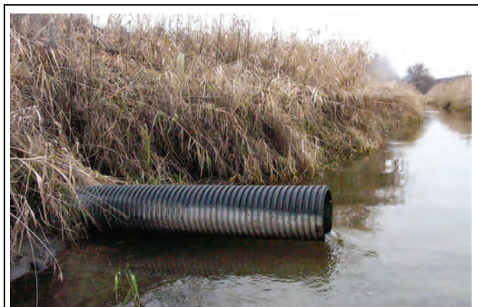
Drain tiles can bypass infiltration and filtration of pollutants by providing a direct pathway to the water and "around" a buffer. This is important to consider in design of a buffer system which integrates with other agricultural practices.
