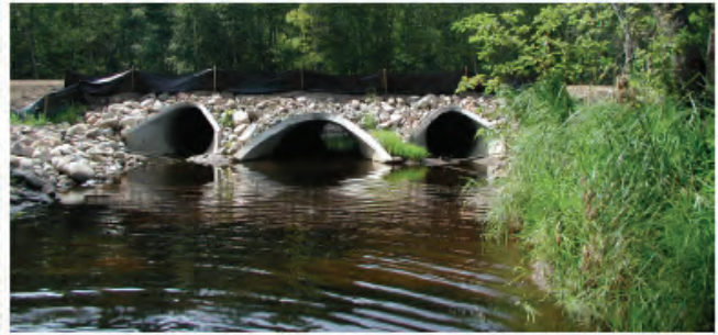
Properly sized and placed culverts.
