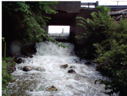
48- LAKE BEULAH DAM/CTH J (RM 1.37)
