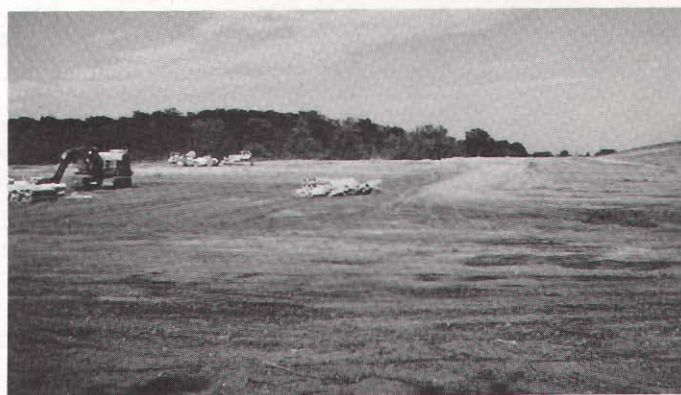
Construction view of the Franklin Industrial Park looking northeast from S. 60th Street south of Ryan Road (STH 100) illustrating the rough grading and sanitary sewer installation.
